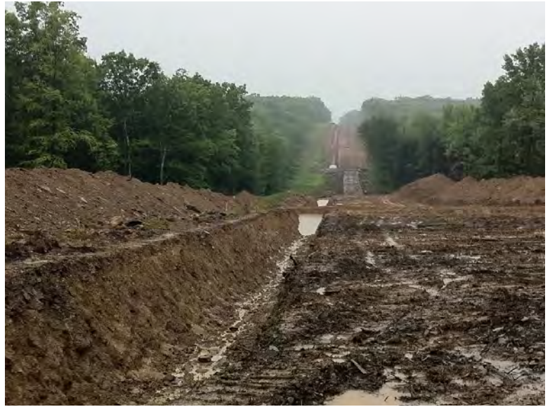
Columbia Gas Pipeline right-of-way carving across Pike County, PA.
