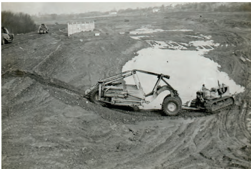
Earth-moving to prepare basins to receive coal sediments. Harold Amster. Used with permission of the Spring Ford Area Historical Society.
