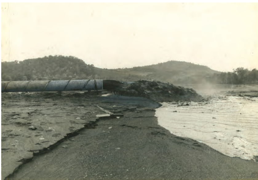
Dredged materials being discharged into the Stoudt's Ferry impounding basin. The Schuylkill River Project Engineers estimated that the slurry was approximately 15 percent solids. This image was included in the Final Report of the Schuylkill River Project Engineers . Used with Permission of the Commonwealth of Pennsylvania, Department of Environmental Protection.
