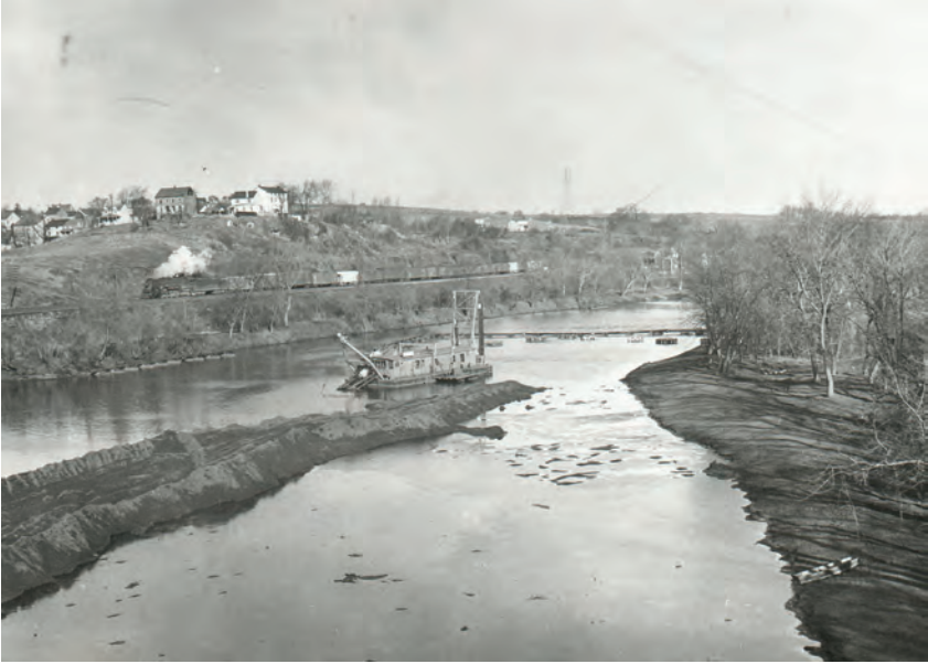
Dredging sediments that have been moved into the River. At lower right, it can be seen that the Schuylkill River is flowing higher than the level of its floodplain. Harold Amster. Used with permission of the Spring Ford Area Historical Society.
