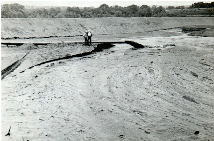
A slurry of water, coal, and sediment is pumped into an impounding basin. The Schuylkill River Project Engineers estimated that the slurry was approximately 15 percent solids. Harold Amster. Used with permission of the Spring Ford Area Historical Society.
