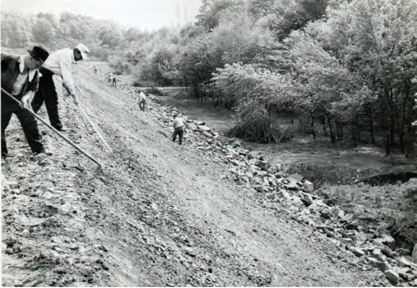
Work on the berm surrounding an impounding basin. The outlet for the impounding basin effluent can be seen at lower right. Harold Amster. Used with permission of the Spring Ford Area Historical Society.
