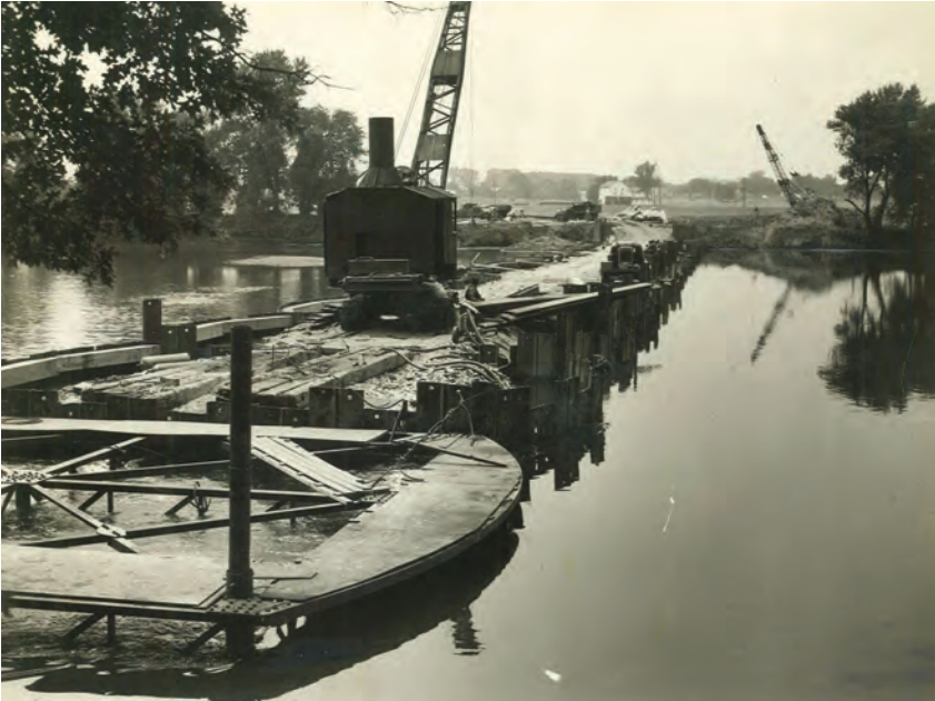
Construction of Linfield temporary dam in 1949. Temporary dams were used to impound water to make it possible for the dredges to operate. This image was included in the Final Report of the Schuylkill River Project Engineers . Used with Permission of the Commonwealth of Pennsylvania, Department of Environmental Protection.
