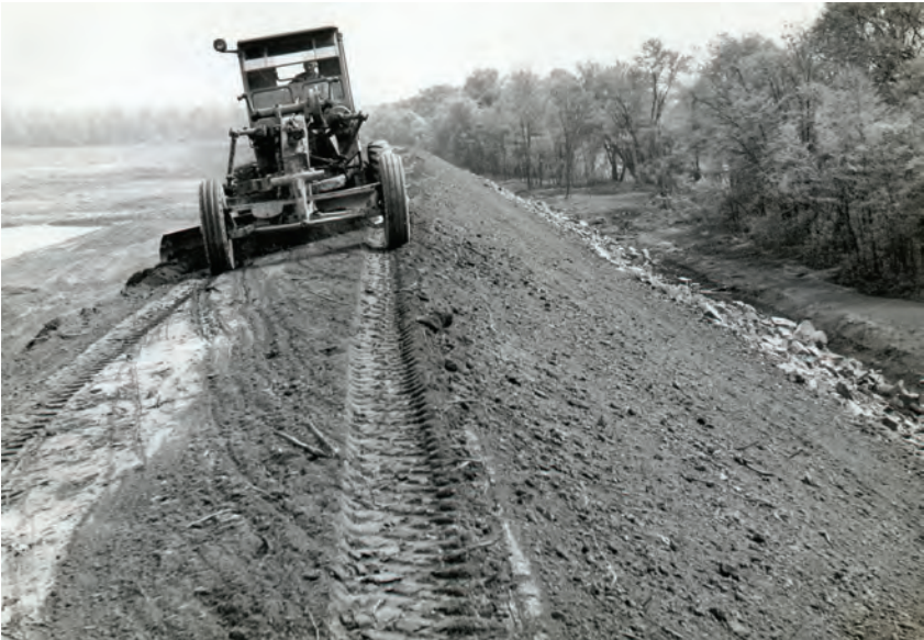
Grading of the top of an impounding basin berm. The impounding basin impact on the river's floodplain can be seen here. The river can be seen through the trees at top right. Harold Amster. Used with permission of the Spring Ford Area Historical Society.
