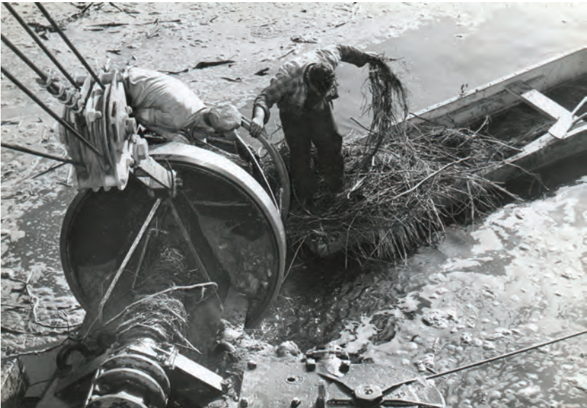
The vegetation bulldozed into the river along with the floodplain coal wastes could clog the cutterhead, intake pipe, or pumps. Other debris in the river that could damage the cutterhead included tires, car fenders, railroad ties, and battered buckets. Harold Amster. Used with permission of the Spring Ford Area Historical Society.
