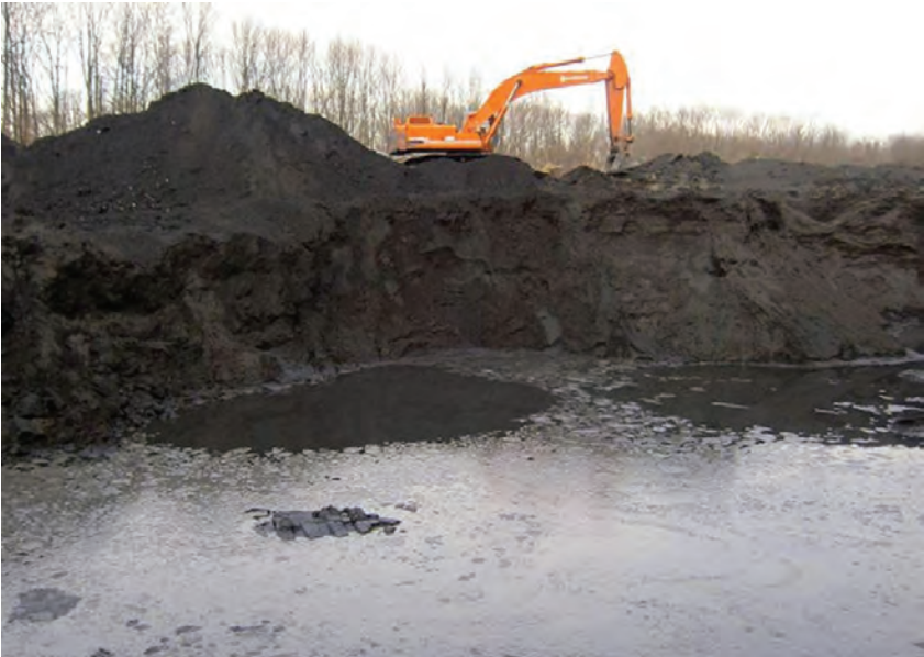
2004 photo showing Stoudt's Ferry Preparation Company excavating dredged sediments from the North Abrams impounding basin to reclaim marketable coal. Used with permission of the Stoudt's Ferry Preparation Company.
