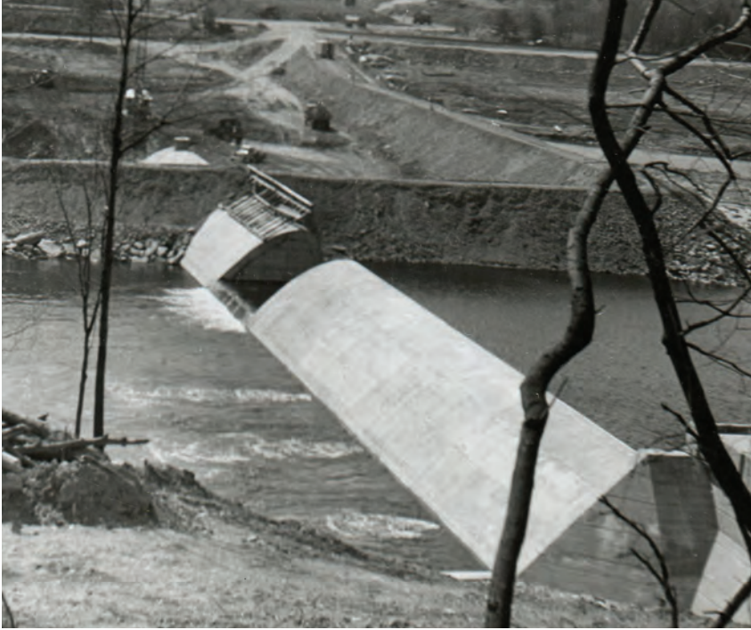
Kernsville Dam under construction. Harold Amster. Used with permission of the Spring Ford Area Historical Society.
