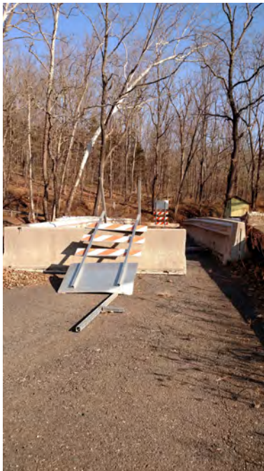
Figure 4 Eastbound view of Headquarters Road Bridge in the area in which the motorcyclist lost control in the 7 May 2006 crash
