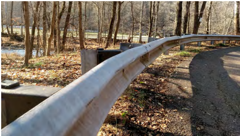
Figure 8 Guardrail along the Headquarters Road curve, showing signs of multiple impacts
