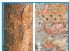
Corroded and pitted casing (Shutterstock). Steel and cement subjected to harsh, corrosive, downhole conditions can degrade in a matter of years, thereby resulting in an explosive, contaminant, and health risk to nearby landowners.
