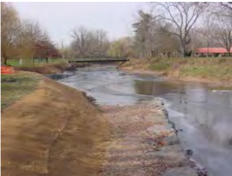
Photo point depicting site after implementation of restoration project that included re-grading and the installation of coir matting and rock vanes. Note footbridge and pavilion in background.
