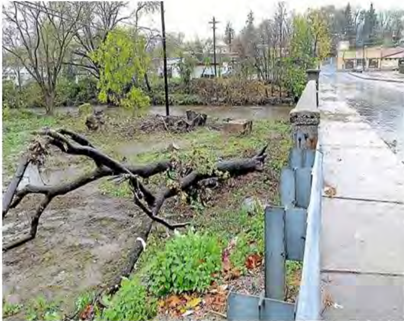
Times file photo The area around the Kerlin Street bridge was among the places in the city damaged by Hurricane Sandy in 2012 .
