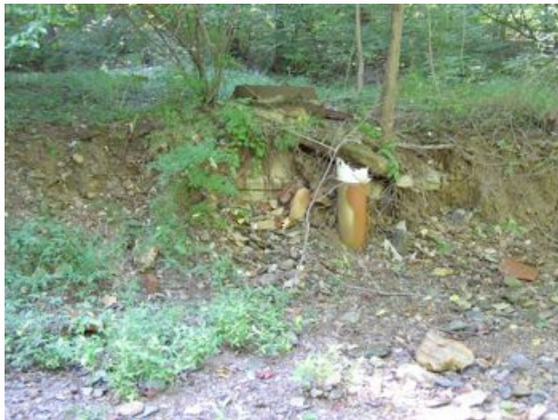
↑ Erosion of sewer line fill in stretch upstream from tunnel under railroad
