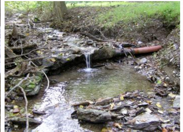
↑ Erosion even in occurs along the sewers the upper headwaters
