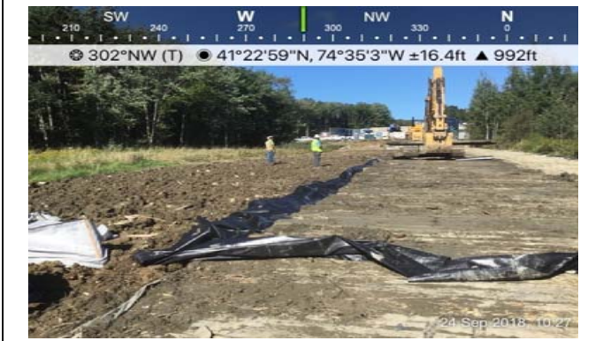
Photograph 7: W-18 (Hugeunot); Contractor placing annual rye seed at crossing as part of the restoration activities.
