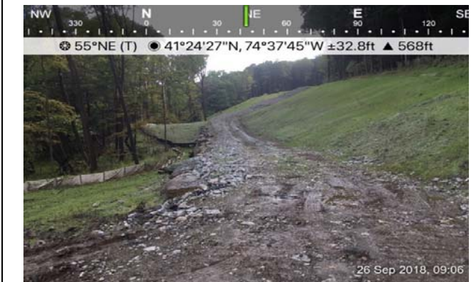
Photograph 3: STA 47+00 (Huguenot); New vegetation growth observed in this area where Contractor recently overseeded.
