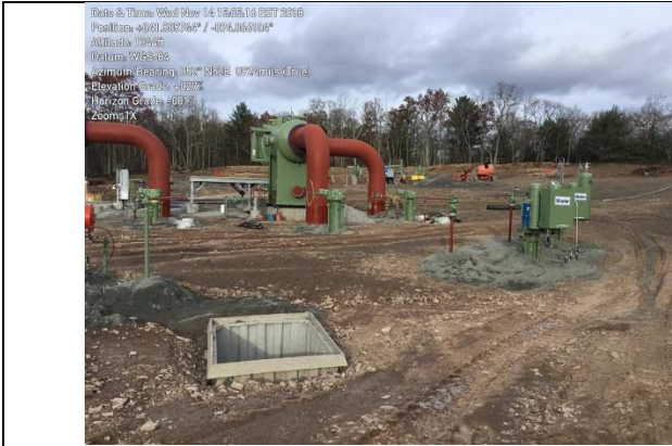
Photograph 1: (Highland) Compressor pad
