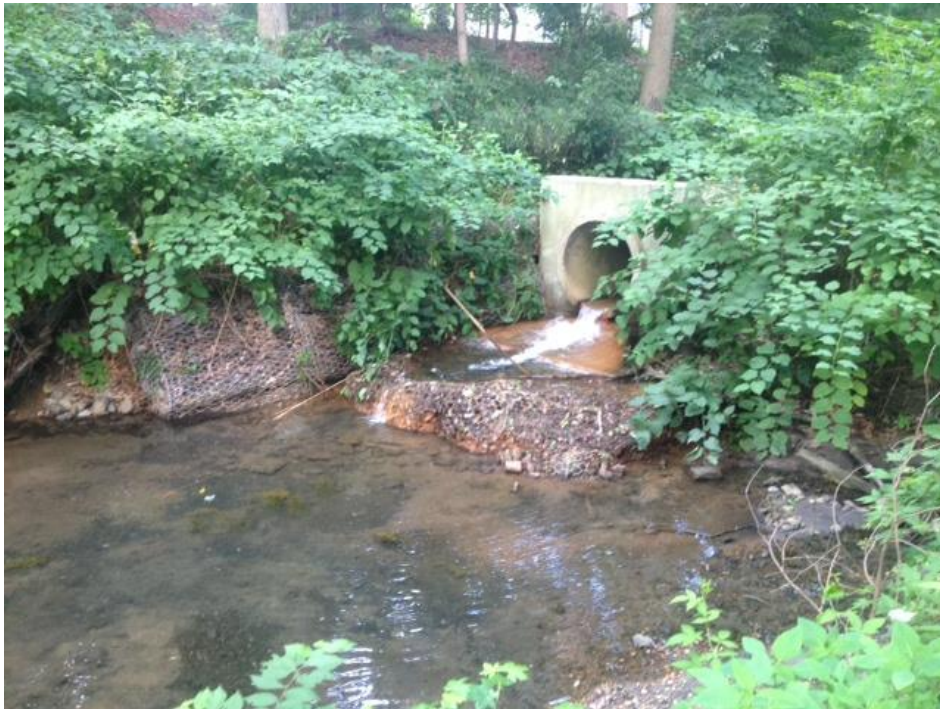
EDISON WOODS OUTFALL PIPE #2 – STREAMBANK REINFORCED AND ARMORED WITH ROCK-FILLED GABION BASKETS DEplete ECOLOGICAL VALUE OF AREA
