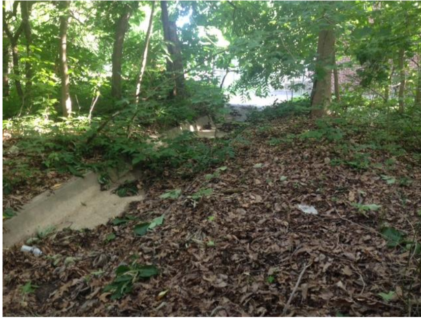
IN EDISON WOODS LOOKING TOWARD CENTER STREET – CONCRETE STORMWATER INLET CHANNELS RUNOFF INTO EDISON WOODS
