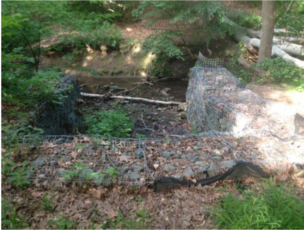
EDISON WOODS OUTFALL #3 – RECEIVES RUNOFF FROM VESPER AVE. OUTFALL REINFORCED AND ARMORED WITH ROCK-FILLED GABION BASKETS. NOTICE LARGE TREE TOPPLED OVER LIKELY THE RESULT OF “DOWN-CUTTING” OF CREEK AND STREAMBANK EROSION
