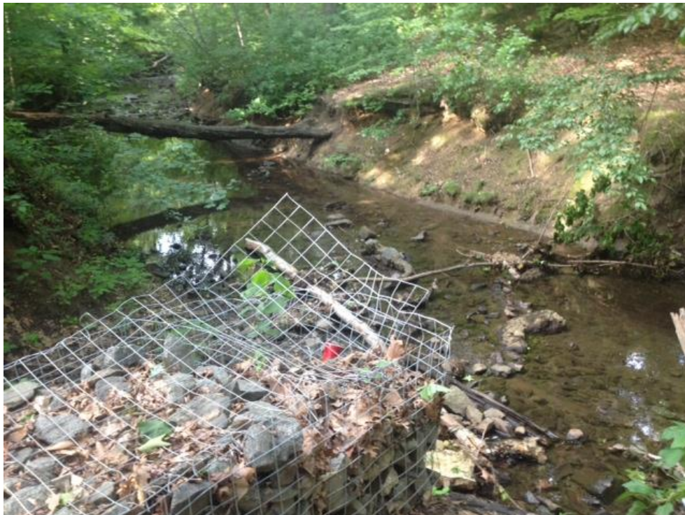
OUTFALL PIPE #3 DAMAGED. NOTE DOWNSTREAM EROSION. ENERGY FROM THREE OUTFALL PIPES ONLY PUSHES ACCELERATED EROSION AND WATER QUALITY DEGRADATION FURTHER DOWN THE CREEK AND THEN INTO THE COOPER RIVER.
