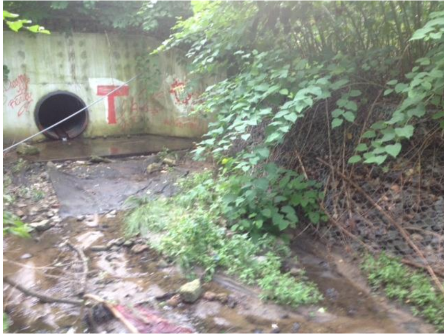
EDISON WOODS OUTFALL PIPE #1 – CONCRETE AND GABION REINFORCEMENT AND ARMORING NECESSARY DUE TO HIGH VOLUMES AND VELOCITY OF STORMWATER. HARD ENGINEERING SUCH AS THIS ONLY MOVES WATERS’ DAMAGING ENERGY FURTHER DOWNSTREAM TO UNPROTECTED SECTIONS
