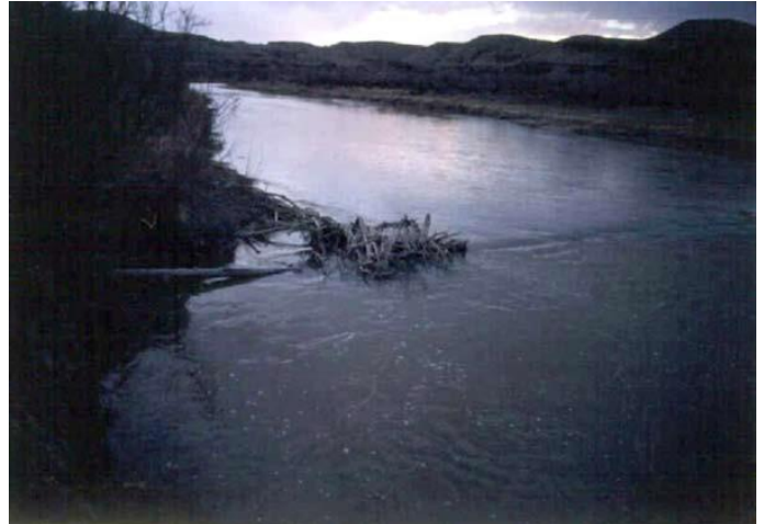
Figure 5: Picture of an exposed pipeline crossing the Green River Utah.
