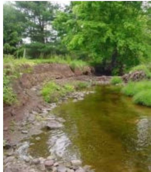
VALLEY CREEK, CHESTER COUNTY, DRN ASSISTED OPEN LAND CONSERVANCY AND RESTORED THIS STREAM REACH WHICH HAD BEEN DEVASTATED BY EROSION.
