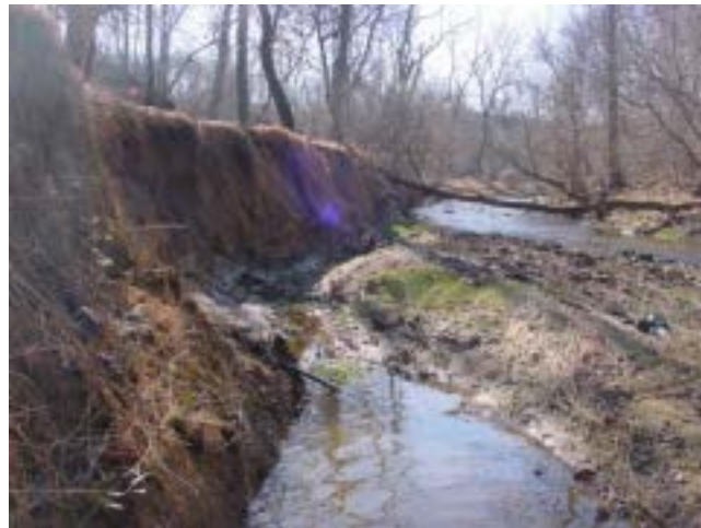
BUCKS COUNTY, PA. BANK EROSION FROM EXCESSIVE RUNOFF IN TINICUM CREEK. THE SEDIMENT FROM THIS BANK RUNS DOWNSTREAM MUDDYING THE WATER, SMOTHERING STREAM BOTTOM HABITAT, AND SUFFOCATING FISH, MUSSELS AND OTHER AQUATIC LIFE.
