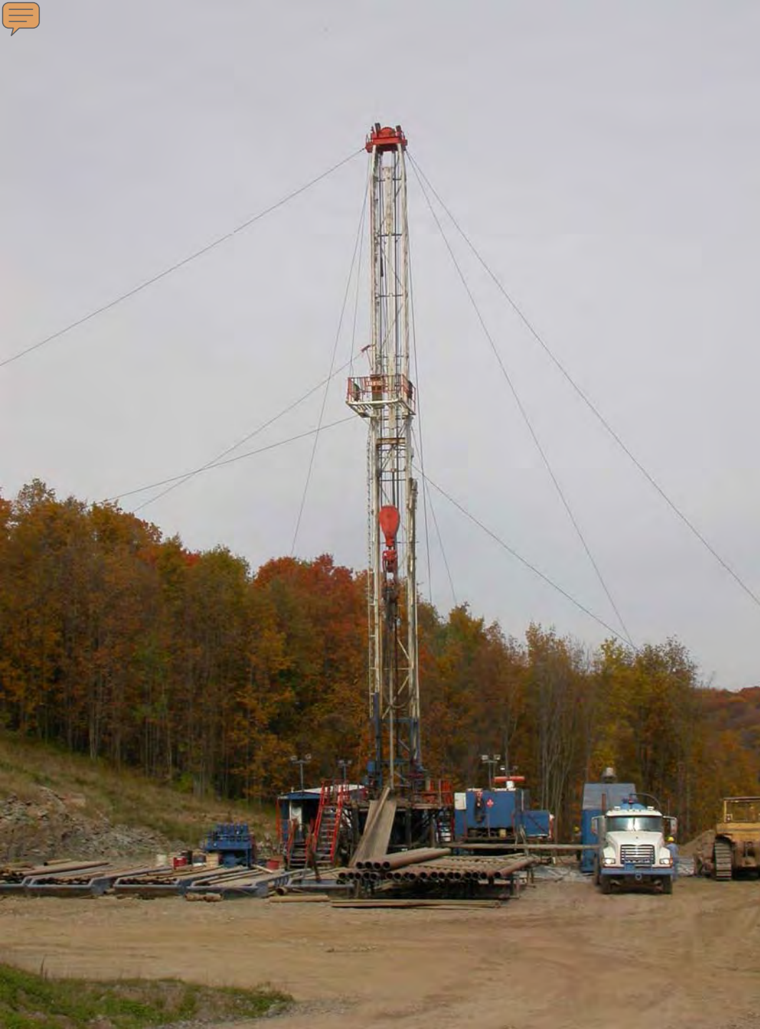
Drilling rig at Dimock Township natural gas well Susquehanna County, PA Cabot Oil and Gas Co.
